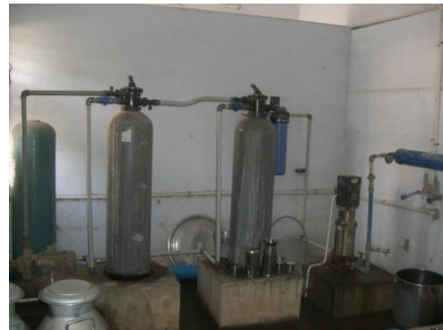
RO Water Plant
